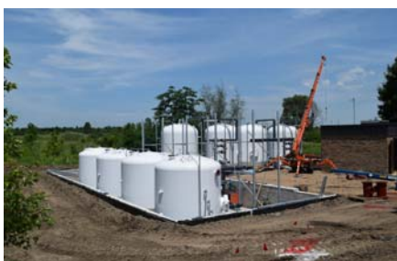
Piping being installed to connect the granular activated carbon tanks and well.
