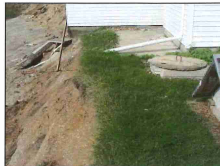
Washed away SSTS in eroded stream bank
